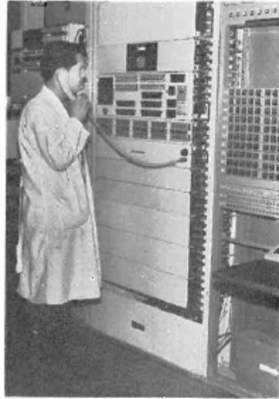
NEW AUTOMATIC EXCHANGE, Numurkah P.O.
