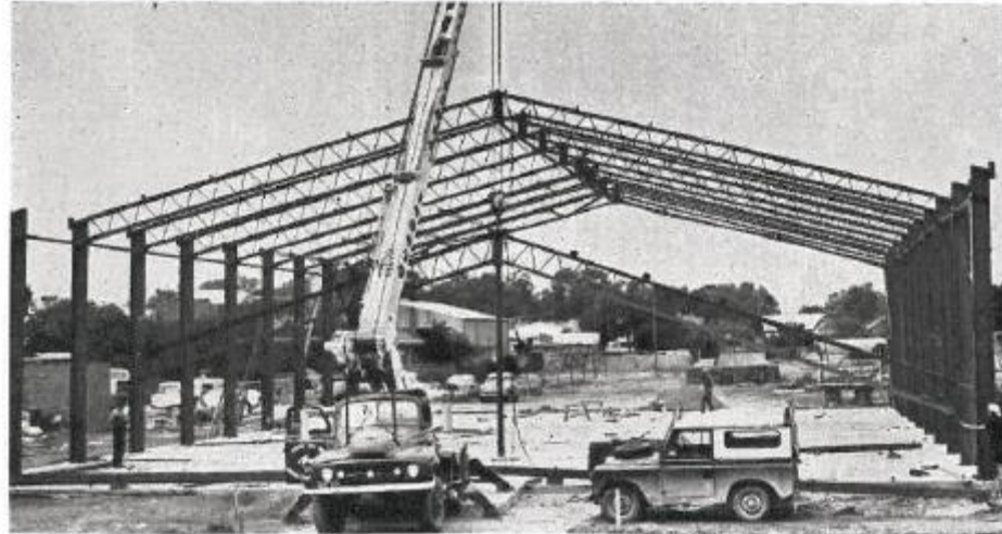
CONSTRUCTION OF NEW STORE FOR PETERSVILLE, McDONALD ST., NUMURKAH A. J. Pumps, Photo.
